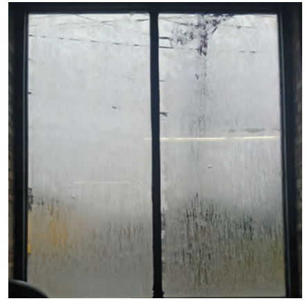
Example of window perf with no lamination in the rain.
