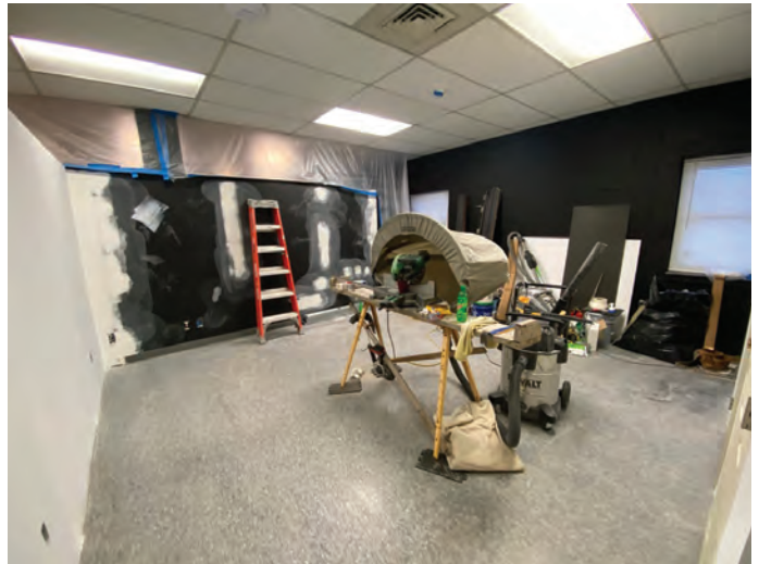
Having the extra space has been a huge help with vinyl installs as well as larger orders for the other processes we offer in the new building.
