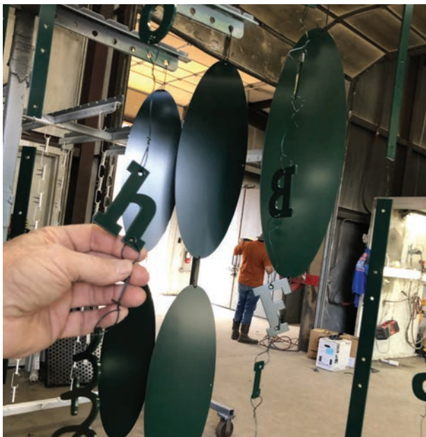
After coating and curing in an oven, all our deep green parts were ready to be installed.
