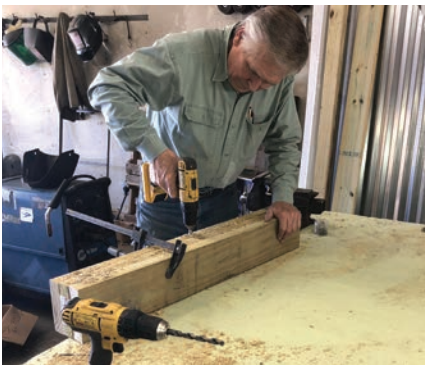
After drill press drilling, holes were reamed out by hand with a slightly larger and longer bit.
