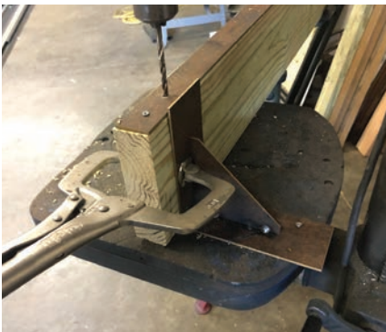
To facilitate permanent threaded rod internal clamps, all boards were drilled on their edges.
