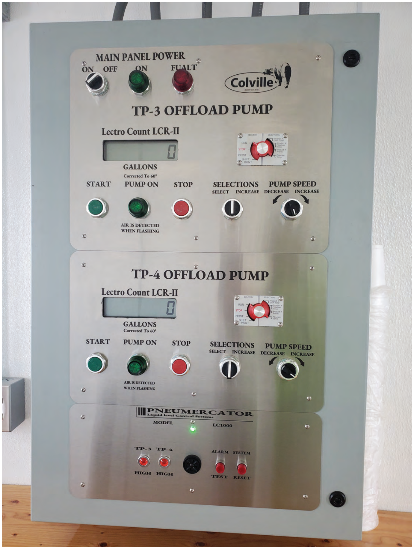
Hatch printed the face plate for a control panel with labels indicating lights, switches, and plates. Hatch uses CerMark metal marking spray paint on metal plates he etches.
