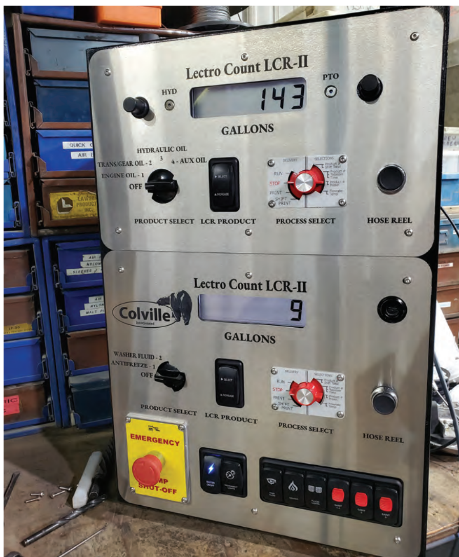
Hatch, project manager of Colville Inc., in Prudhoe Bay, Alaska, built a control panel inside a lube truck and printed the labels to indicate the purpose of the panel's individual switches and controls. (All images courtesy Heber Hatch)
