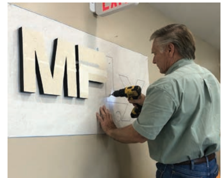
In the field, the patterns are carefully set in place, and small 3/16"-diameter holes are drilled.
