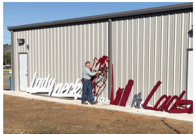
Before beginning the install, all parts are spread out in handy fashion along the building's wall.
