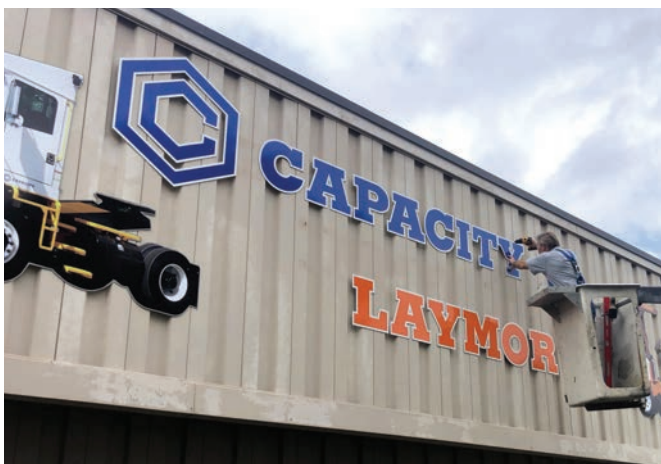
The install was a one-man job, as all the parts were light and easy to work with.
