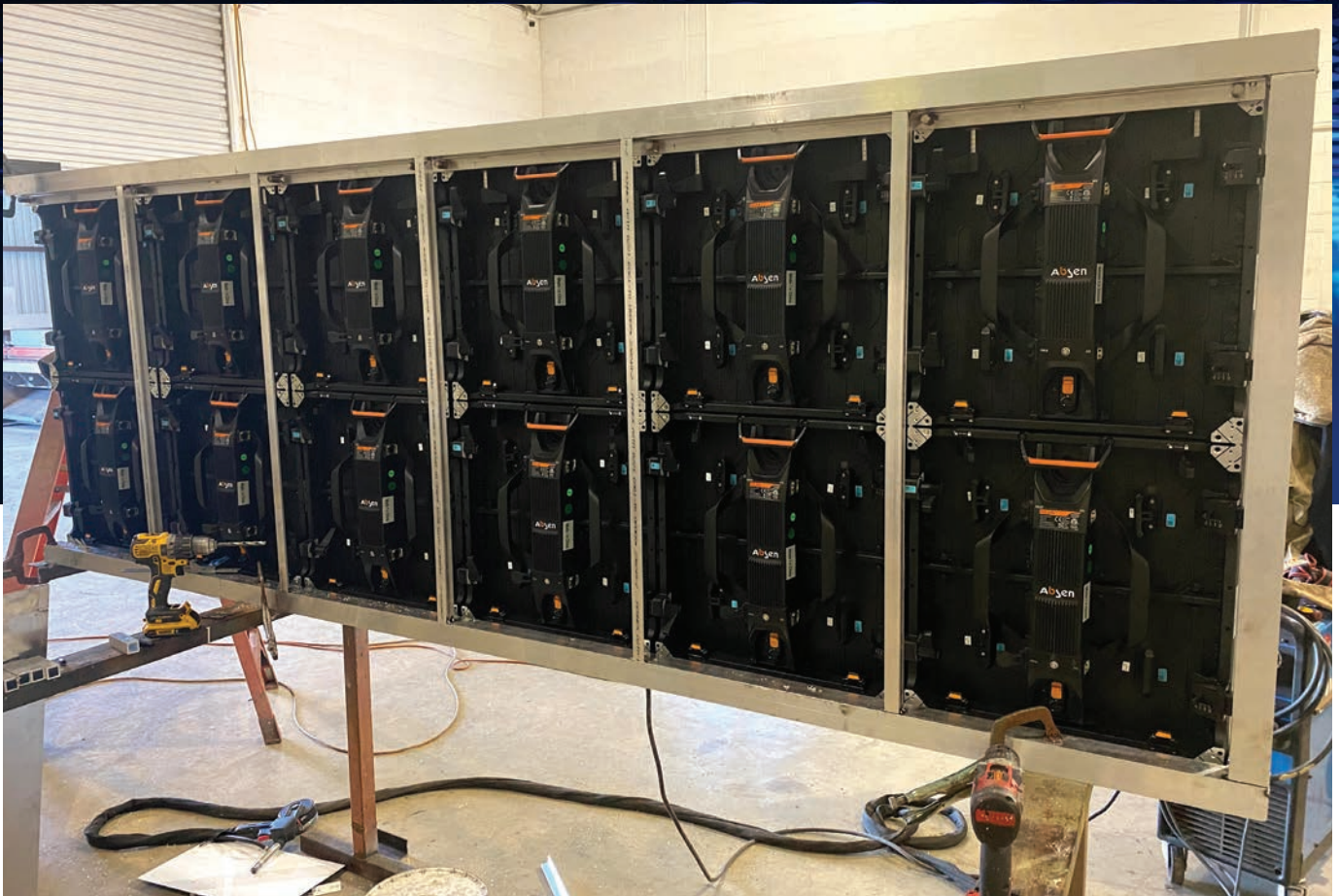
Here you can see the backs of the display units after they were installed.
